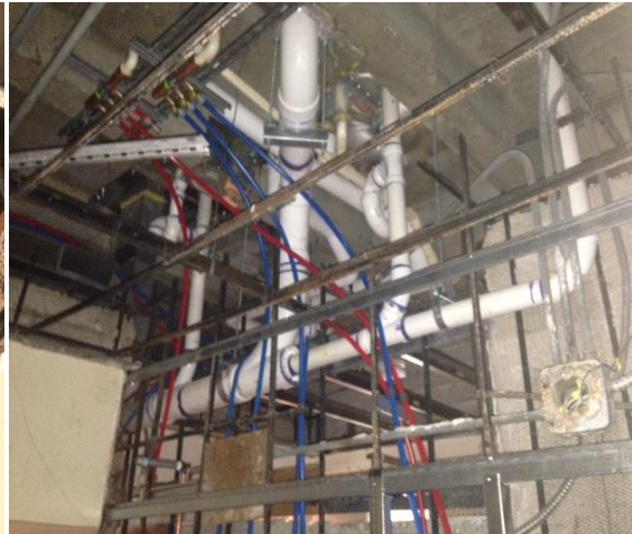
New Pex piping – J-wing
