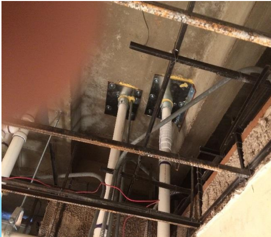
Firestop b/w floors – J-wing
